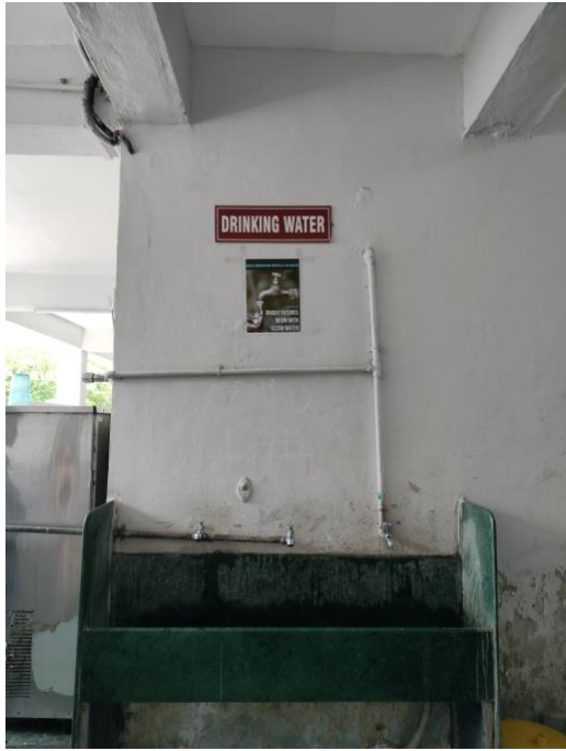
DRINKING WATER FACILITY
